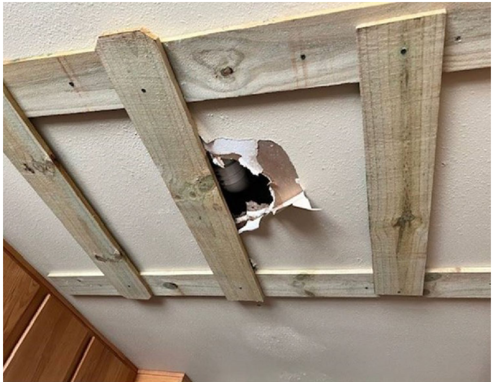
Figure 1: Ceiling with Hole Braced with Fence Pickets in Privatized Home on Naval Air Station Key West
