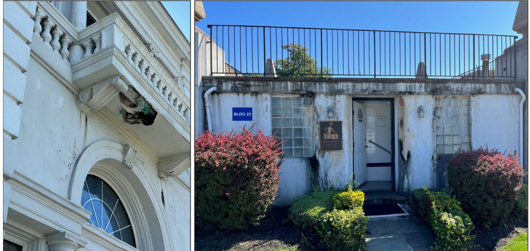
Decaying facade on Wiley Hall administration building.
