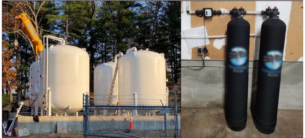
Figure 6: Examples of Granular Activated Carbon (GAC) Filtration in Large and Small Public Water Systems
