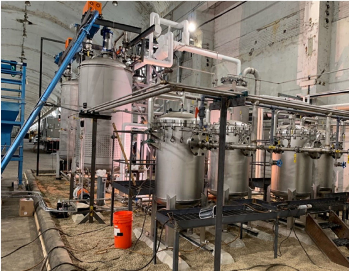
Figure 5: A pilot-scale facility in Pennsylvania for rare earth element extraction from coal ash
