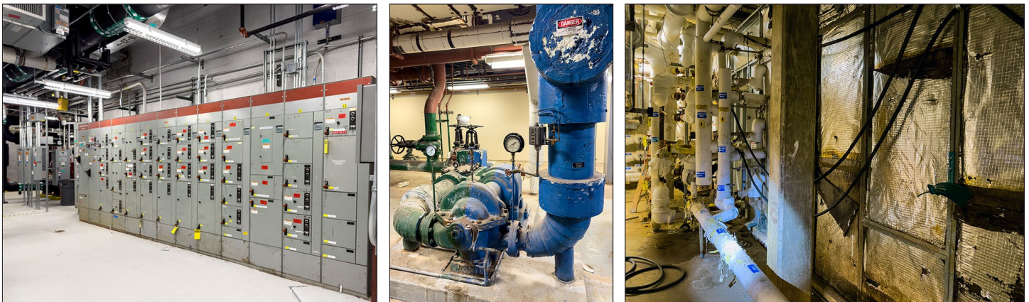
Figure 8: Brookhaven National Laboratory: Physical Plant Equipment Slated for Capital Replacement but Included in Deferred Maintenance and Repair Estimates
