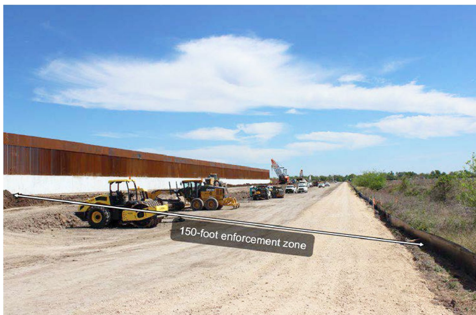
Figure 2: Border Barrier and Enforcement Zone under Construction in Rio Grande Valley Sector
