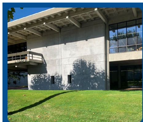
A shear wall that is part of a seismic retrofit of a university library
