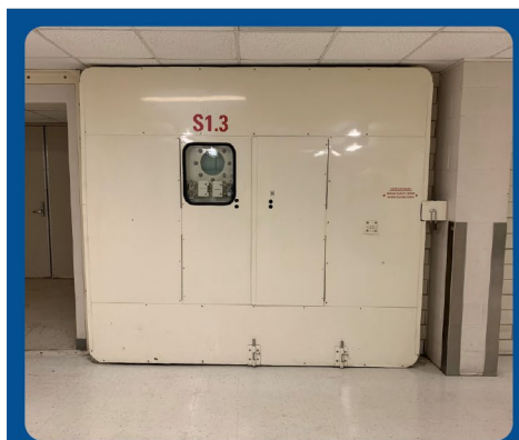
Watertight enclosure to prevent floodwater damage
