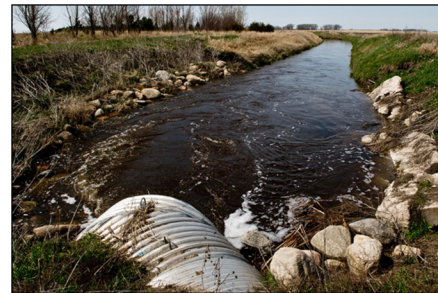
Rocks and an angled culvert help prevent bank erosion in North Dakota.
