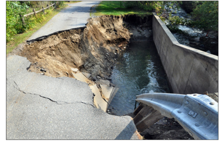
In 2011 tropical storm Irene caved in many roads after dropping more than 11 inches of rain. This caused floods, which did extensive damage to infrastructure in Vermont.
