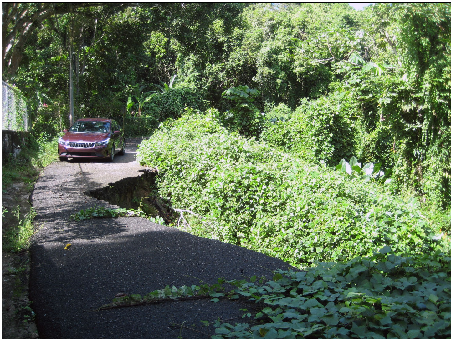
Figure 4: Collapsed Segment of Road Near Maricao, Puerto Rico, September 2018
