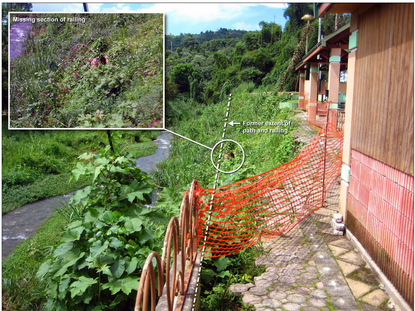
Figure 5: Missing Rail in Public Space Along River's Edge, Maricao, Puerto Rico, September 2018
