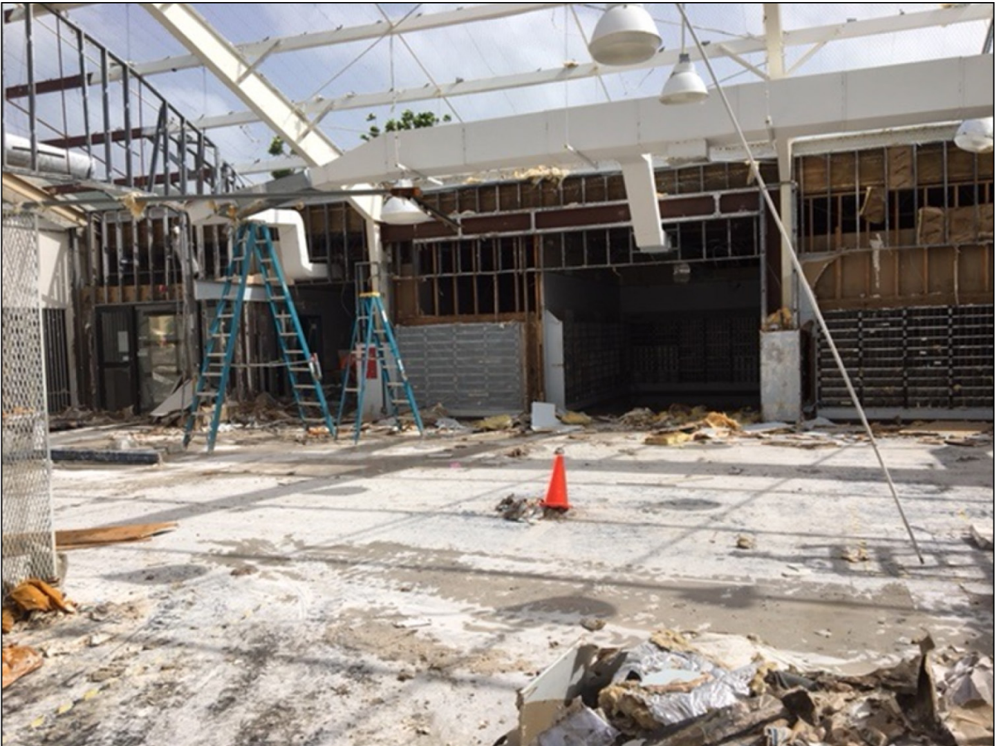
Figure 4: U.S. Postal Service Facility Damaged during Hurricane Maria
