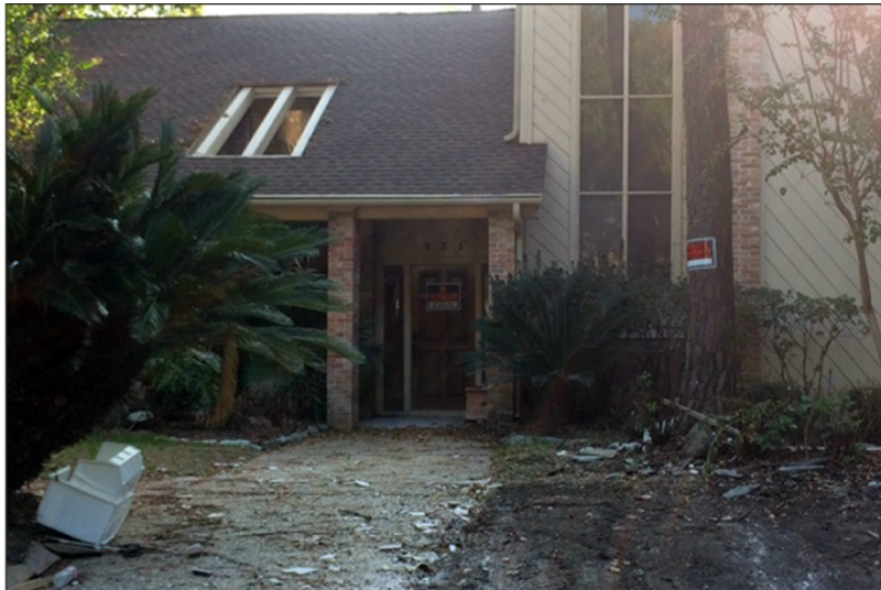
Storm damaged home in Harris, County, Texas.
