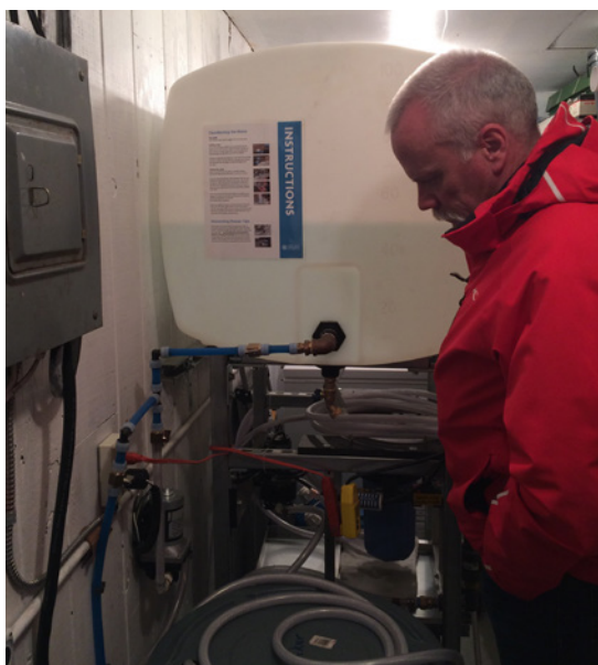
Analyst inspects a pilot water system in a home in Kivalina, Alaska, during a review of Indian water infrastructure.
