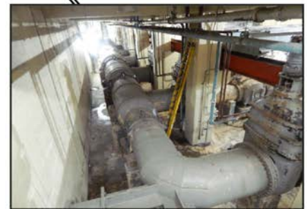
Main pumps and discharge pipe
