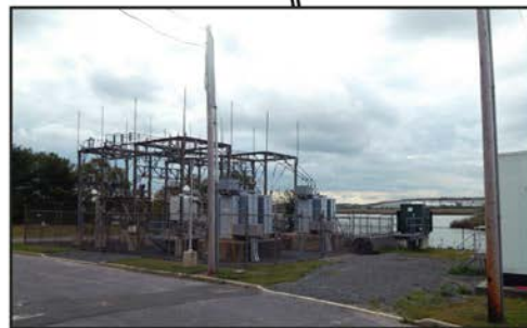
Pumping station power grid
