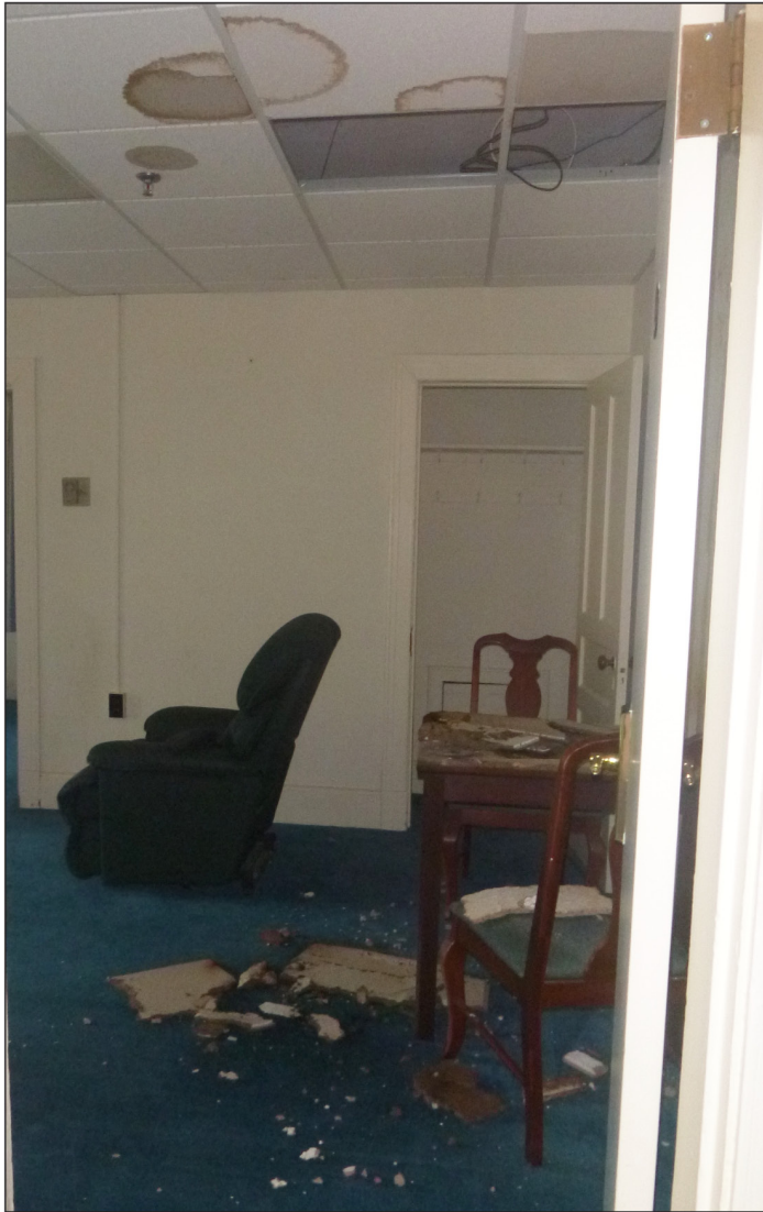
Figure 8: Example of Property Needing Repairs at Fort Monmouth, New Jersey
