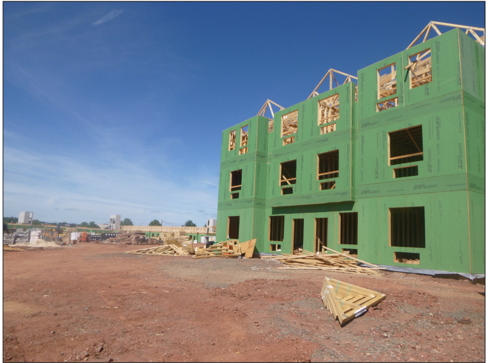
Figure 10: A Mixed-Use Development under Construction at Sergeant J.W. Kilmer U.S. Army Reserve Center, Edison, New Jersey
