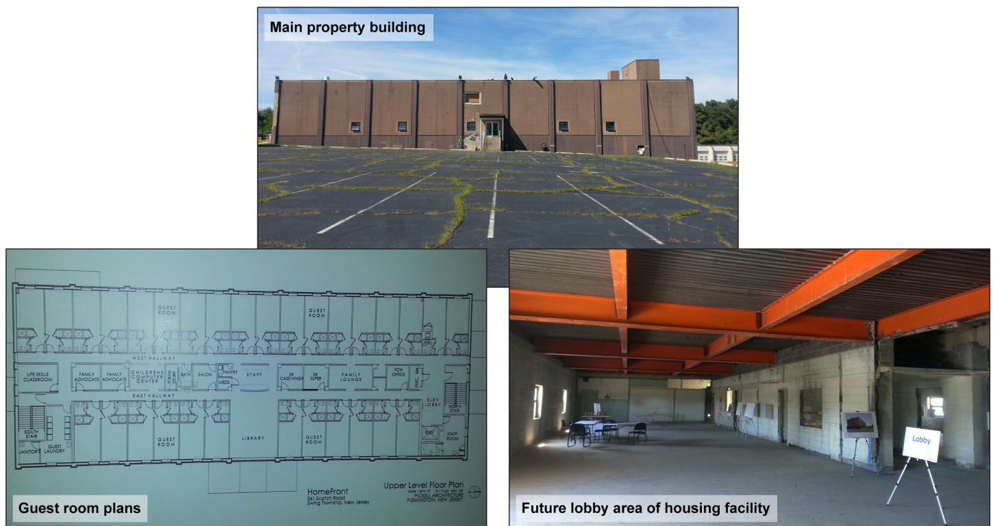
Figure 5: Renovations at the Inspector/Instructor Facility at West Trenton Marine Corps Reserve Center
