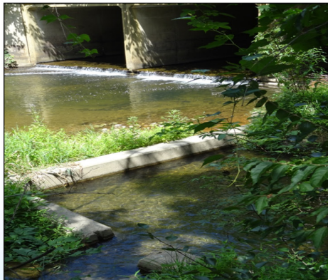
USDA: It was unclear to USDA officials what purpose this retaining area, marked as a dam, fulfills at Beltsville, Maryland.
