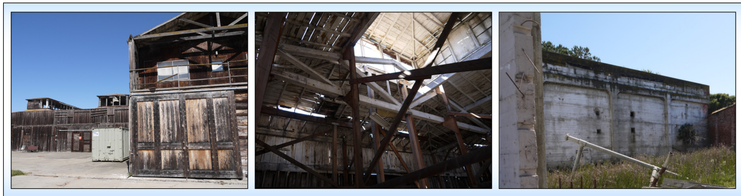
Figure 7: Examples of the Condition of Interior’s Fish and Wildlife Service’s Historic Cannery at Don Edwards San Francisco National Wildlife Refuge in California
