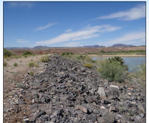
Interior: Headgate Rock Dam is a diversion dam to irrigate Indian lands in California.
