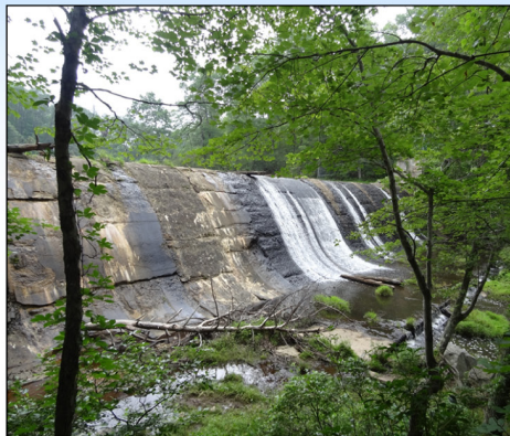
Interior: Prince William Forest Park Camp 5 Dam – built to create a swimming area in Virginia.
