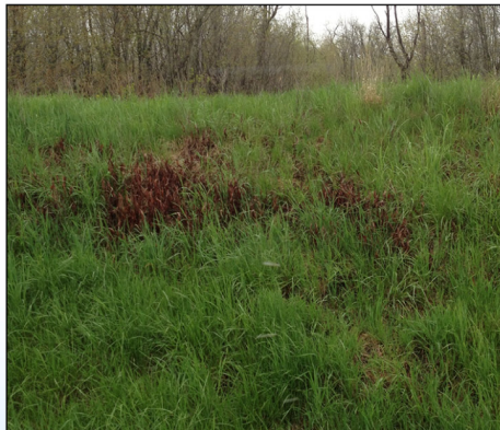
DOE: Earthen dam built to retain storm water runoff at Fermi National Accelerator Laboratory in Illinois.
