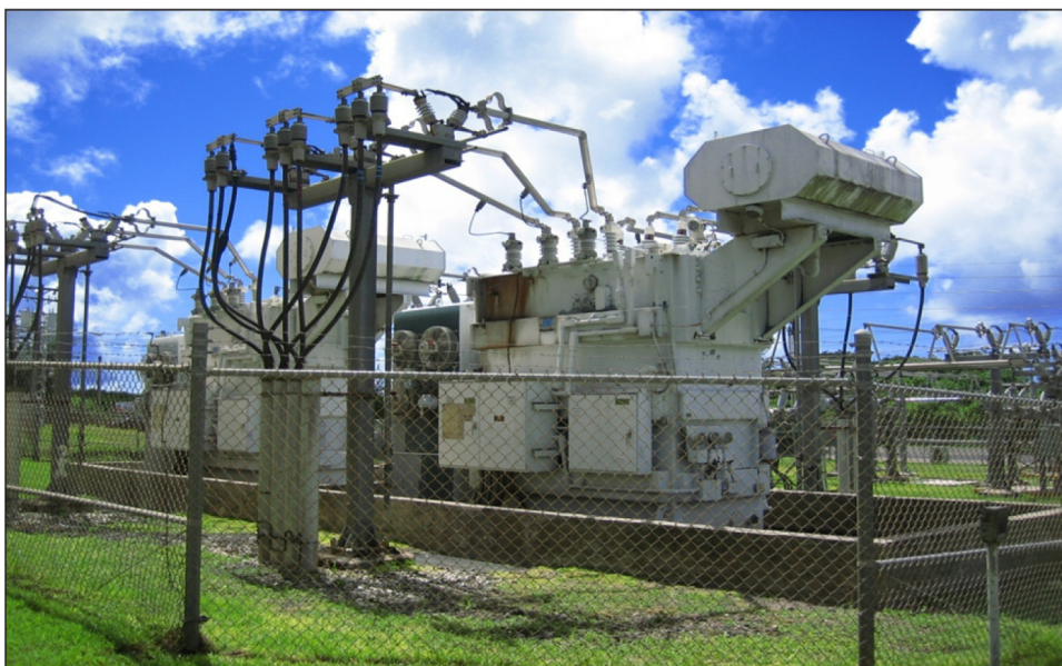
Figure 3: Harmon Annex Power Station
