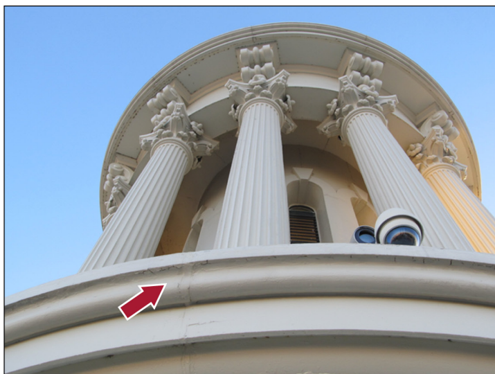
Figure 3: Damage to Capitol Dome, Outside Left, Inside Right (2013 Photographs)
