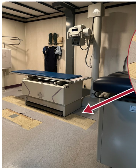
Missing floor tiles at an X-ray room at Lodge Grass Health Clinic, Montana. New flooring was needed before new equipment could be used. Officials reported that this flooring was later repaired in December 2022 following our visit.
