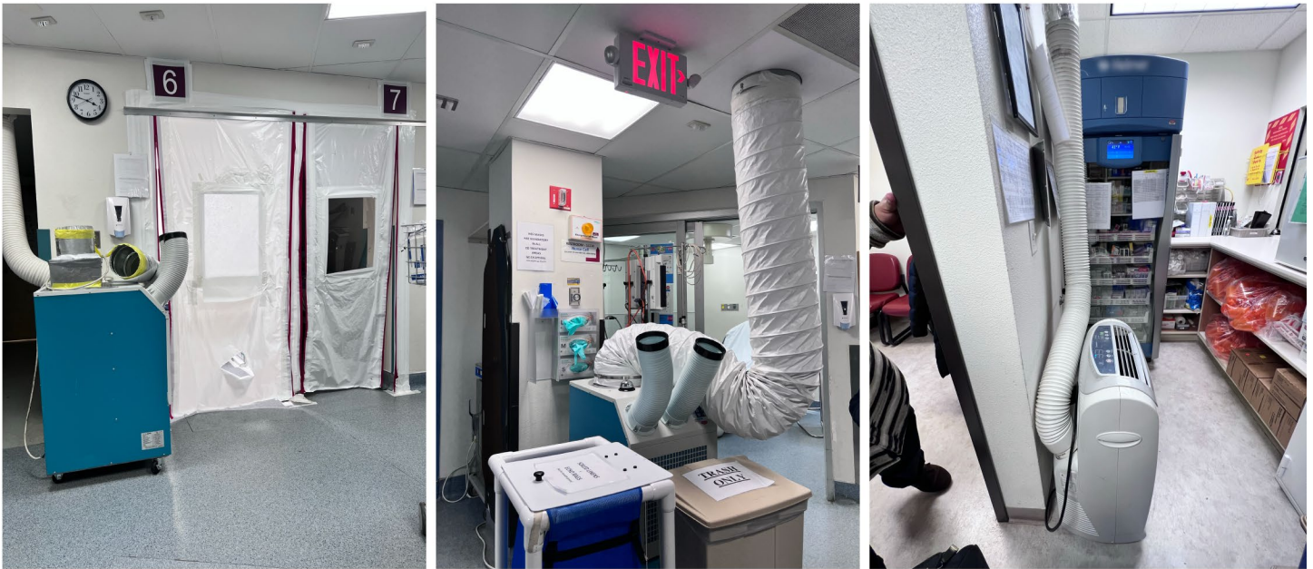
Work-arounds developed by IHS facilities staff in the Navajo area to address issues such as air flow and temperature control.
