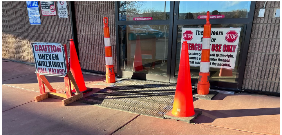
"Caution: Uneven walkway. Fall Hazard." - Sign posted at the entrance to the emergency department at the IHS Crownpoint Comprehensive Health Care Facility.
