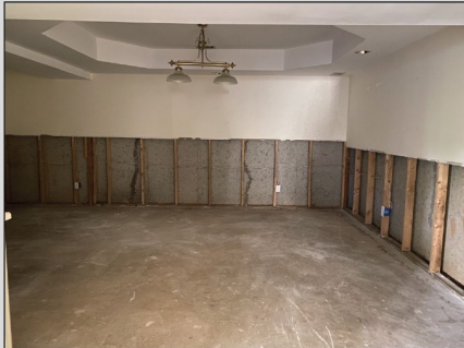
Water and mold damage to walls.
