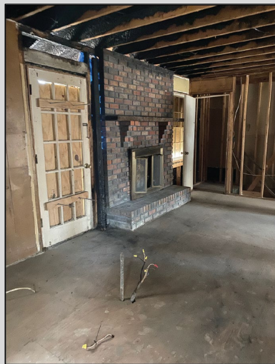
Exposed wiring and missing drywall.
