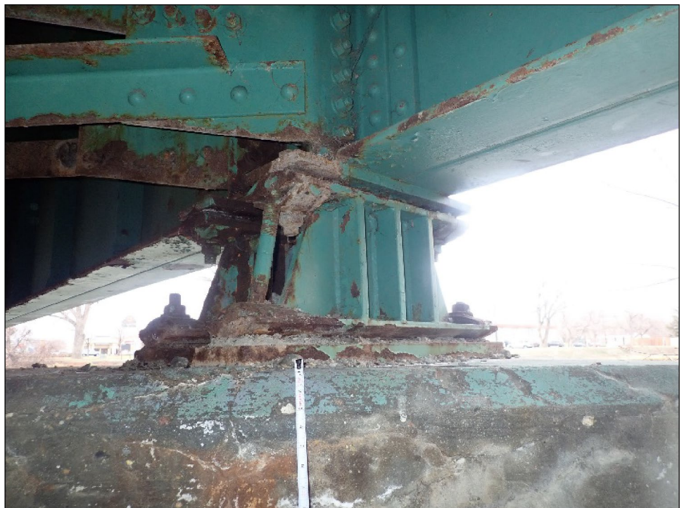
Figure 14: Photo of Corrosion on a National Highway System Wyoming Bridge
