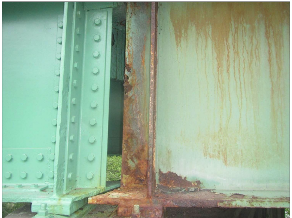
Figure 12: Photo of Corrosion on a National Highway System Rhode Island Bridge
