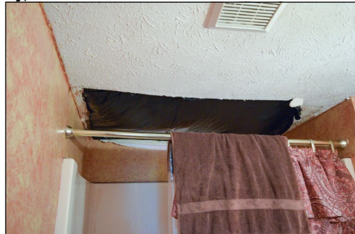
A survivor patches a leak in her home with a trash bag nine months after Hurricane Michael caused a tree to fall on her house.
