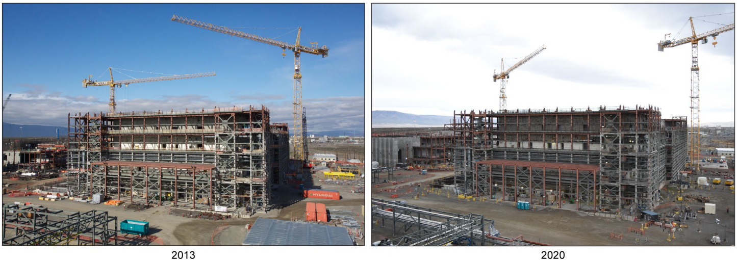
Figure 1: The Partially Constructed Pretreatment Facility at the Hanford Waste Treatment and Immobilization Plant
