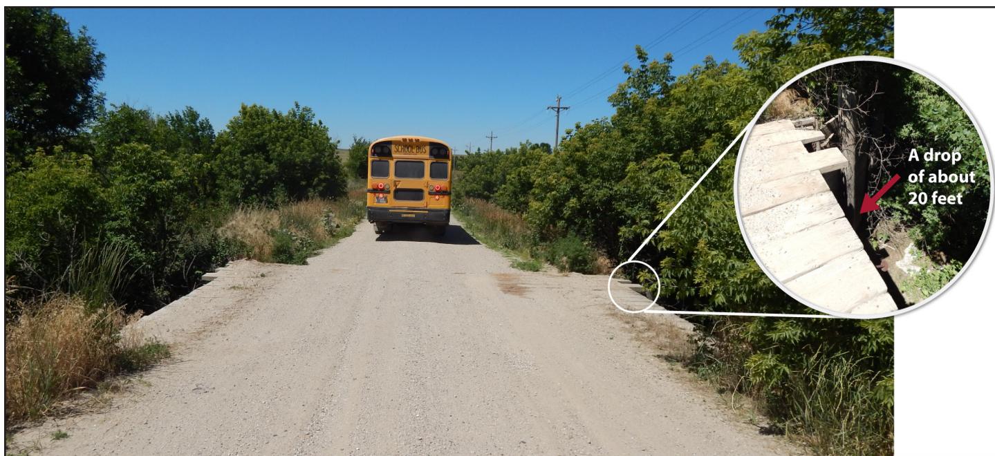
Figure 9: School Bus Route Traversing a Wooden Bridge on the Pine Ridge Reservation
