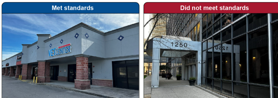
Figure 5: Examples of Readjustment Counseling Service (RCS) Inspection Findings Related to Exterior Condition
