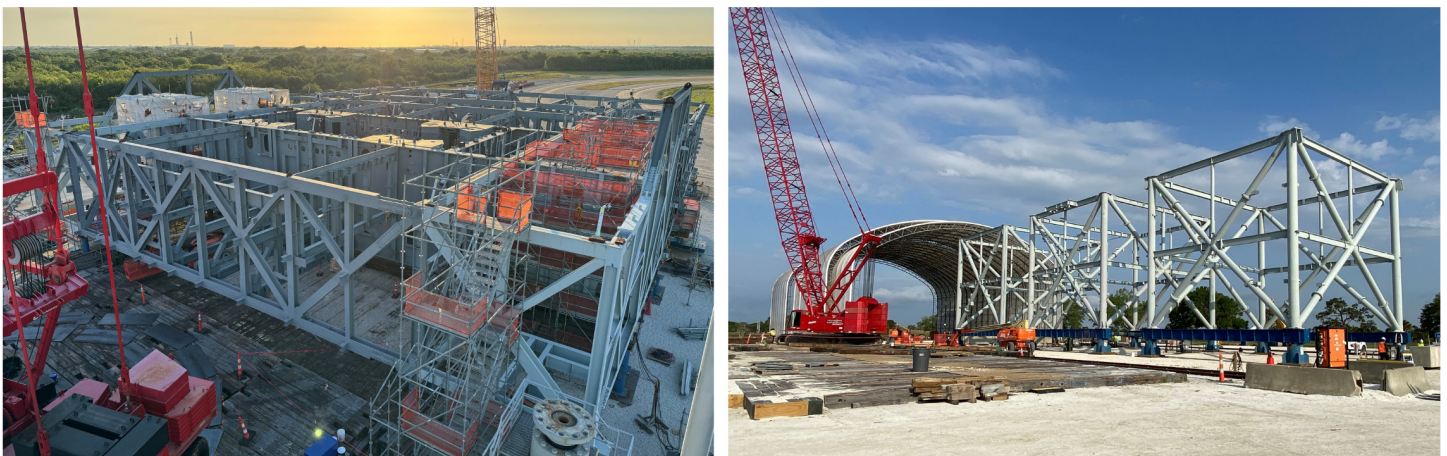
Figure 6: Photos of Mobile Launcher 2 Base and Tower Construction Sites as of July 2024
