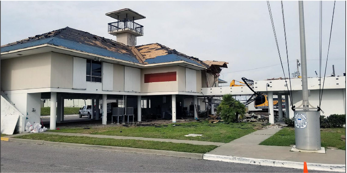
Figure 5: Damage at Station Port Aransas in Texas, Resulting from Hurricane Harvey in 2017
