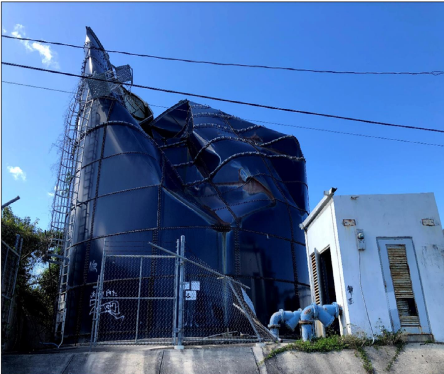
Damaged water tank from winds of Hurricane Maria observed in February 2020
