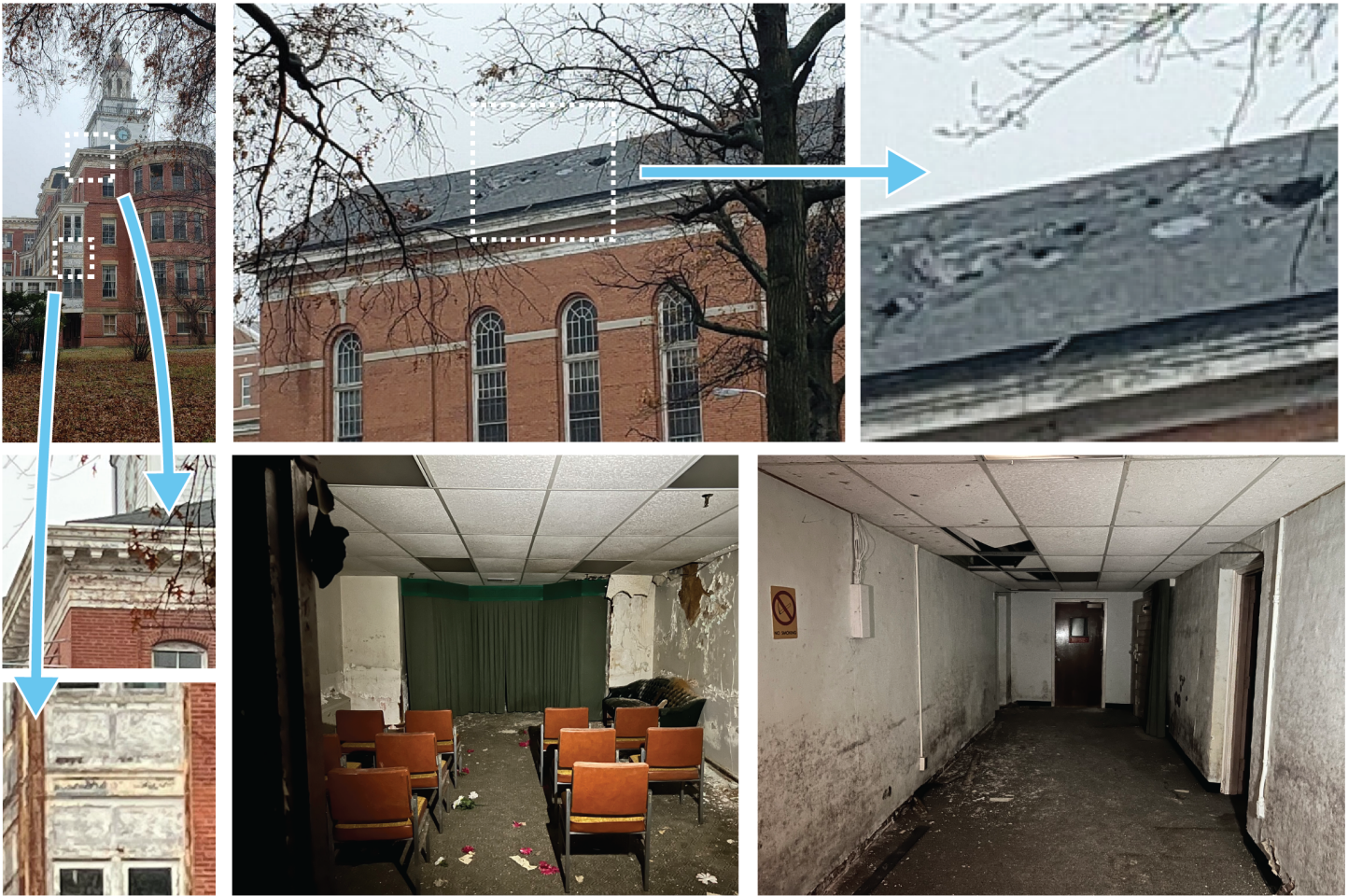
Figure 6: Examples of Exterior and Interior Building Damage at the Armed Forces Retirement Home in Washington, D.C.
