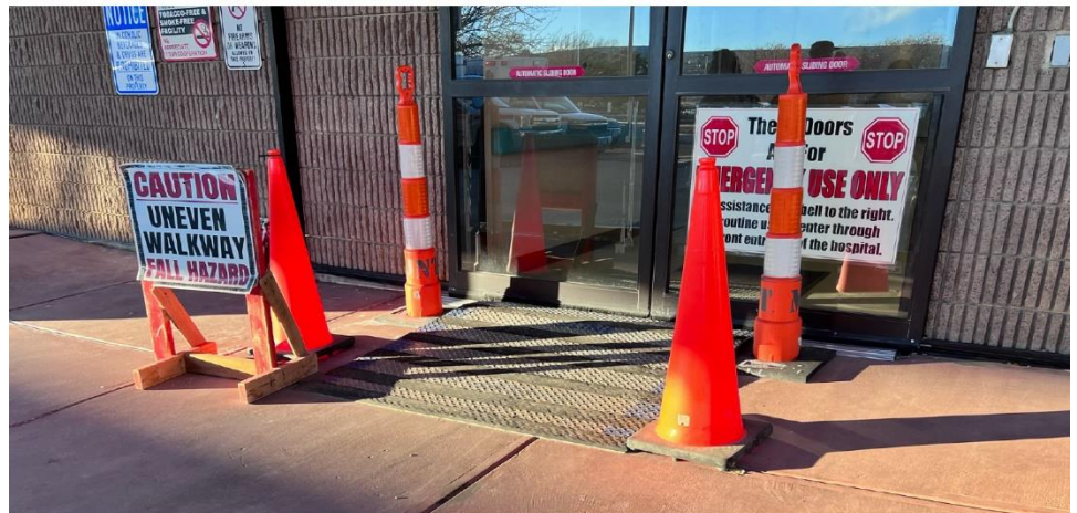
Figure 14: Photo of a Fall Hazard at the Emergency Department Entrance of a Navajo Area Indian Health Service (IHS) Facility
