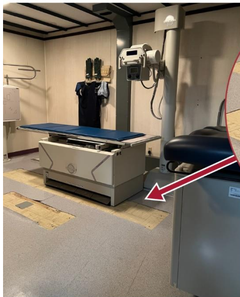
Missing floor tiles at an X-ray room at Lodge Grass Health Clinic, Montana. New flooring was needed before new equipment could be used. Officials reported that this flooring was later repaired in December 2022 following our visit.
