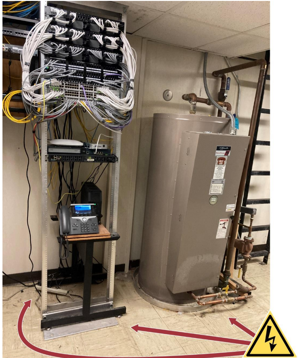
Figure 6: Hazardously Located Facility Equipment at the Indian Health Service Lodge Grass Health Clinic Due to Lack of Space
