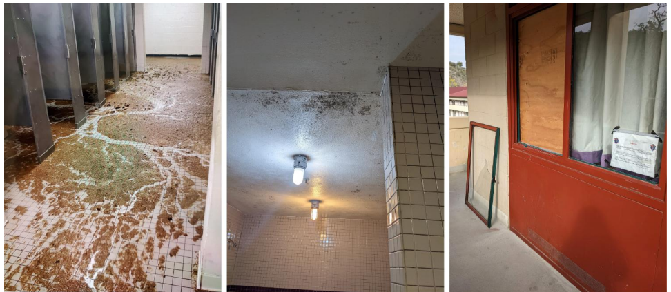
Figure 1: Potentially Serious Health and Safety Risks at GAO Site Visit Locations
