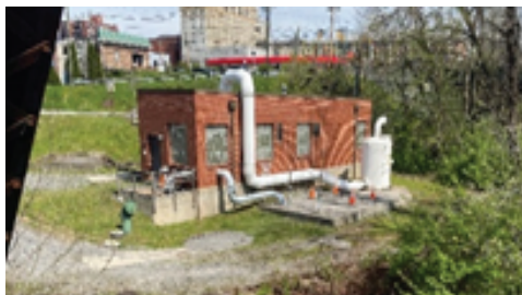
Deckers Creek Pump Station Source: GAO photo. | GAO-23-105285
