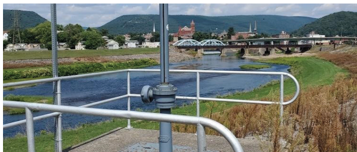
CSO outfall looking upstream at Potomac River, Cumberland, Maryland. Source: City of Cumberland, Maryland | GAO-23-105285
