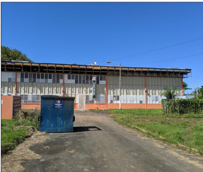
School with internal mold and water damages caused by Hurricane Maria observed in March 2019.
