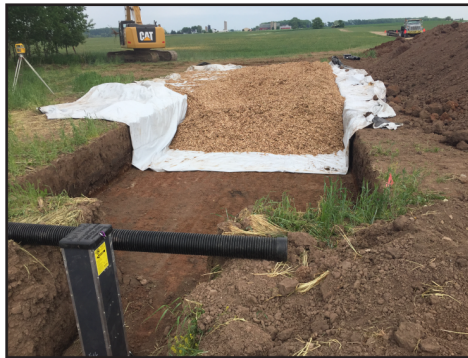
Bioreactor being filled with wood chips
