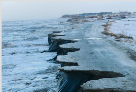
Damage to Shishmaref sanitation road
