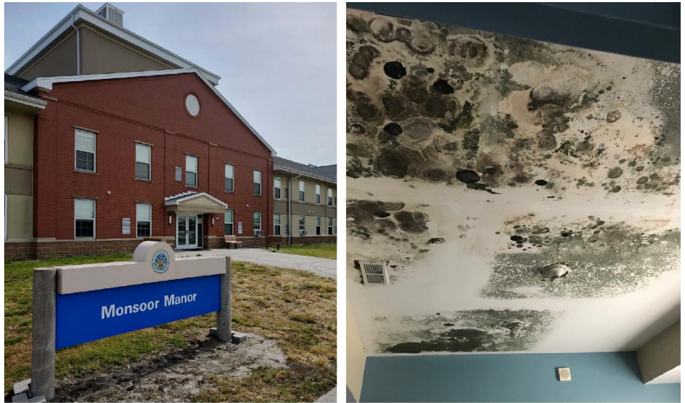
Figure 6: Naval Station Norfolk, Virginia, Living Quarters with a Mold-Affected Room
