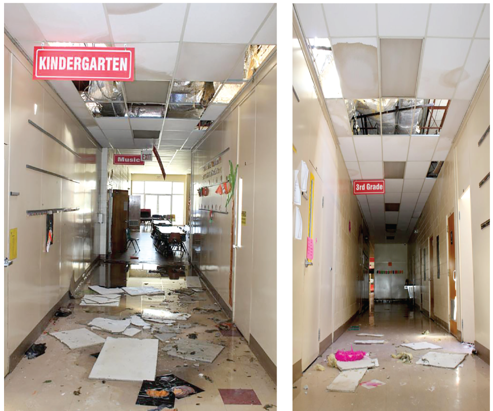
Figure 7: School Facilities Damaged by Hurricane Michael in Florida
