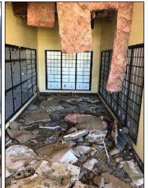
Collapsed ceiling and insulation debris at Panama City-Northside Station Post Office, Panama City, Florida
