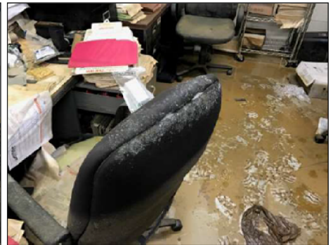
Mold on chair at Bear Creek Vehicle Maintenance Facility, Houston, Texas
