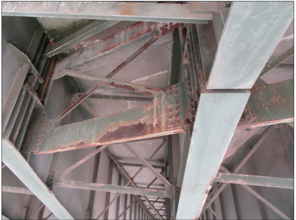
Figure 10: Photo of Corrosion on a National Highway System Kansas Bridge
