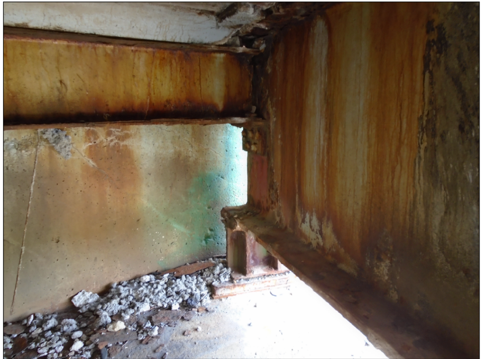
Figure 8: Photo of Corrosion on a National Highway System's Illinois Bridge
