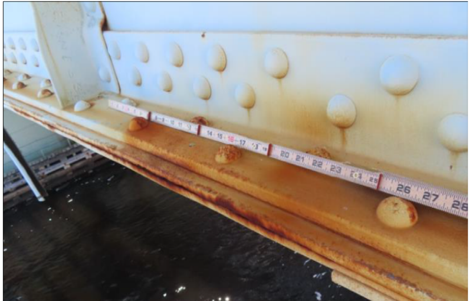
Figure 6: Photo of Corrosion on a National Highway System Florida Bridge
