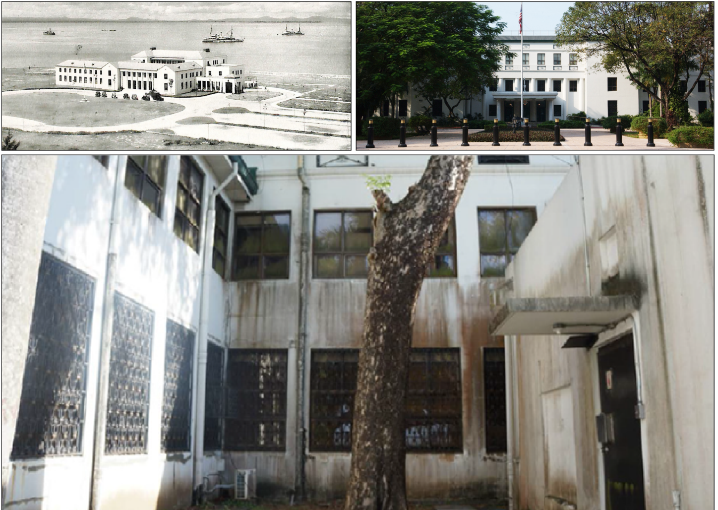
Figure 9: U.S. Embassy Manila, Philippines – Chancery Office Building: Top Left (in 1940); Top Right (in 2019); and Bottom - Chancery Courtyard Showing Maintenance Issues, Including Mold and Water Damage
