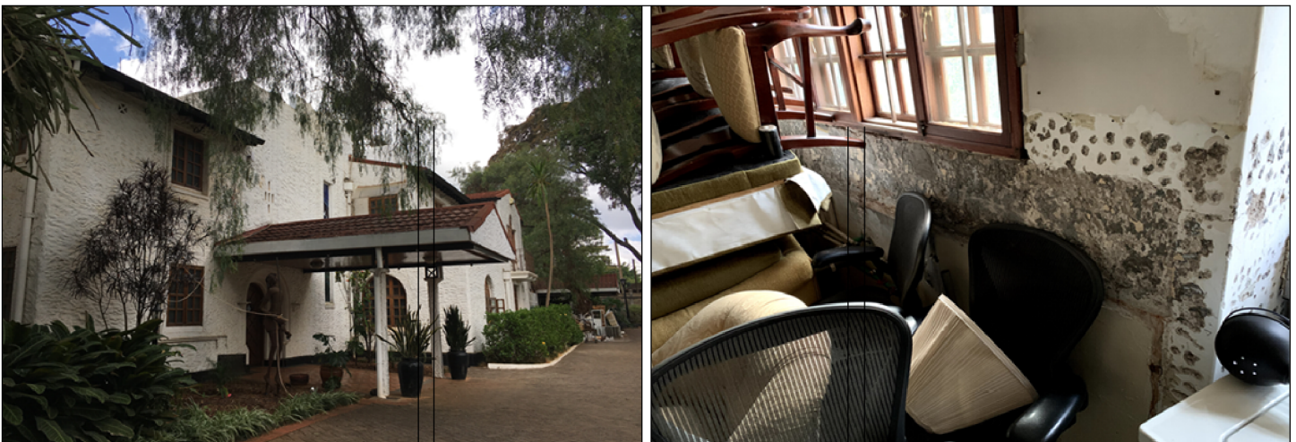
Figure 11: U.S. Ambassadorial Residence - Nairobi, Kenya. Built in 1935. Left - Covered Entryway That Needs to Be Rebuilt. Right – the Kitchen Area Now Demolished and Used to Store Furniture Until State Determines Whether to Rehab the Residence or Replace It Entirely
