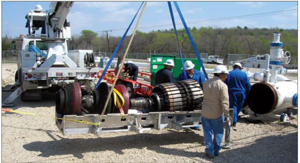
Figure 2: In-Line Inspection Tool Being Placed in a Launch Point on a Pipeline
