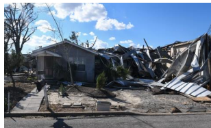
Tyndall Air Force Base, Florida (2018) Damage from Hurricane Michael
