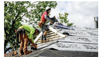
Fort Carson, Colorado (2017 / 2018) Damage from wind and hail storms
