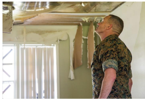
Marine Corps Base Camp Lejeune, North Carolina (2018) Damage from Hurricane Florence a
