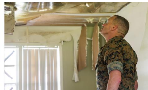
Marine Corps Base Camp Lejeune, North Carolina (2018) Damage from Hurricane Florence*
