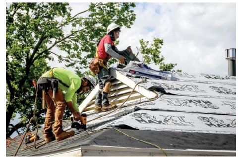
Fort Carson, Colorado (2017 / 2018) Damage from wind and hail storms
