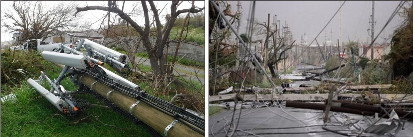
Figure 2: Examples of Damage Caused by Hurricanes Irma and Maria, September 2017
