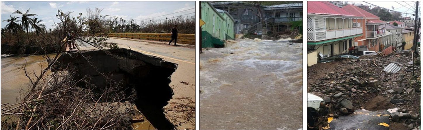
Figure 3: Examples of Damaged Roads in Puerto Rico and the U.S. Virgin Islands, September 2017
