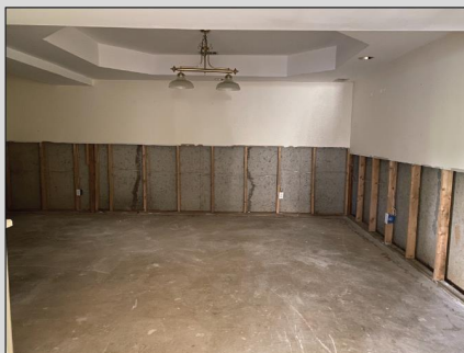
Water and mold damage to walls.
