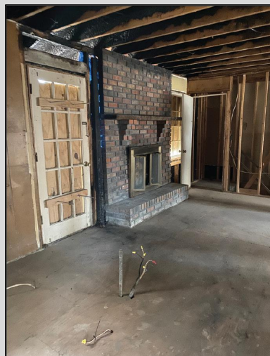
Exposed wiring and missing drywall.
