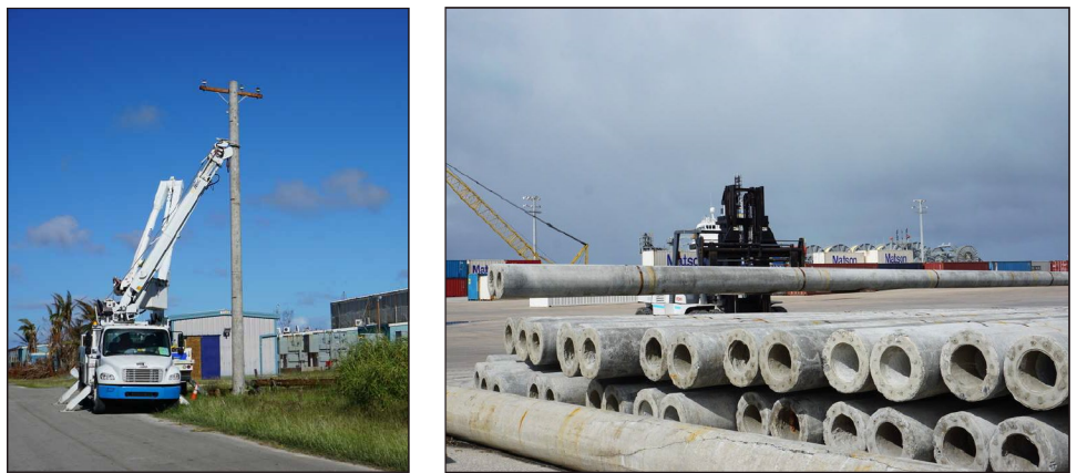
Figure 14: Concrete Utility Poles Installed in the Commonwealth of the Northern Mariana Islands as a Hazard Mitigation Initiative
