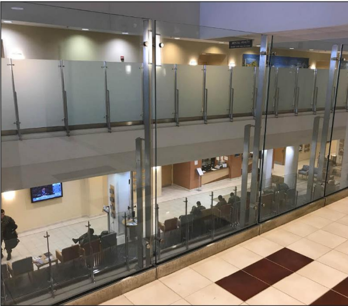
Heightened barriers added at a medical center to prevent attempts to jump into the open atrium.
