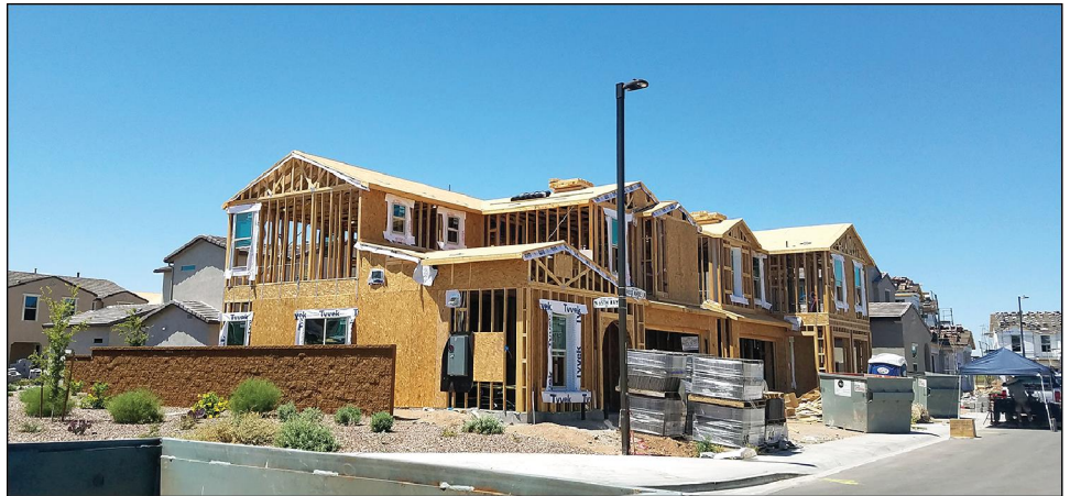
Figure 12: Housing Units Being Constructed by Company that Subcontracts with an H-2B Employer in Maricopa County, Arizona
