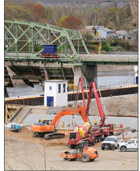
Infrastructure on Lock-9 of the Erie Canal system on the Mohawk River is being repaired for flood control systems.
