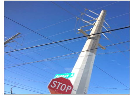
Reinforced power line poles.
