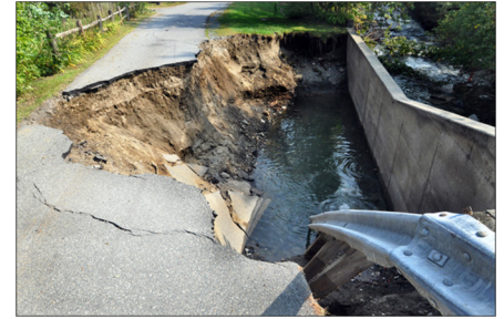
In 2011 tropical storm Irene caved in many roads after dropping more than 11 inches of rain. This caused floods, which did extensive damage to infrastructure in Vermont.
