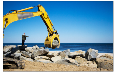
6,000-pound boulders being stacked to build an 18-foot barrier to reinforce the Bay's Head, New Jersey, sea wall as part of Hurricane Sandy relief efforts.
