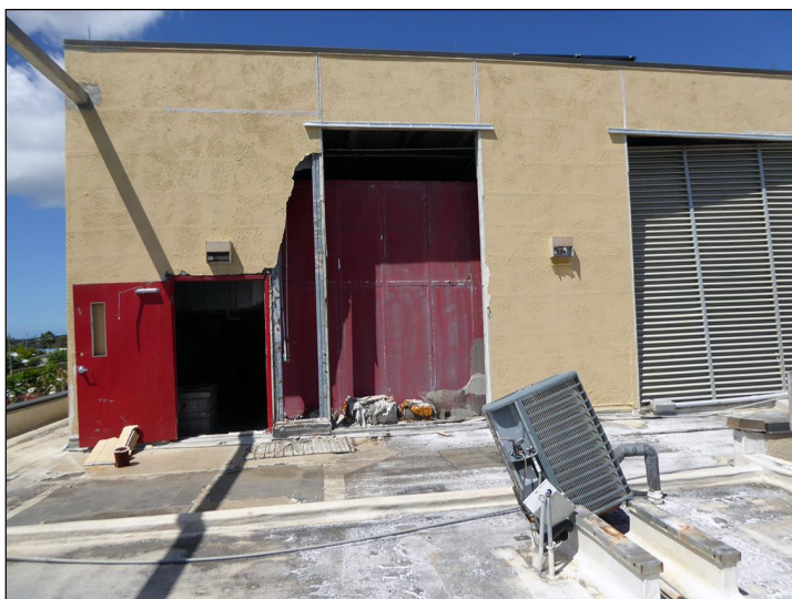
Damaged structure and ventilation system of the Governor Juan F. Luis Hospital and Medical Center in St. Croix, U.S. Virgin Islands.
