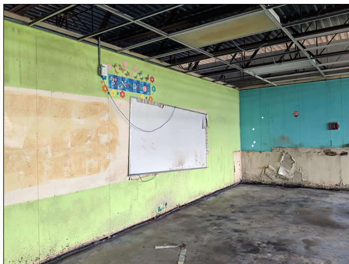
Classroom with mold on the walls and water damage on the walls at the Berwind Intermediate School in San Juan, Puerto Rico.
