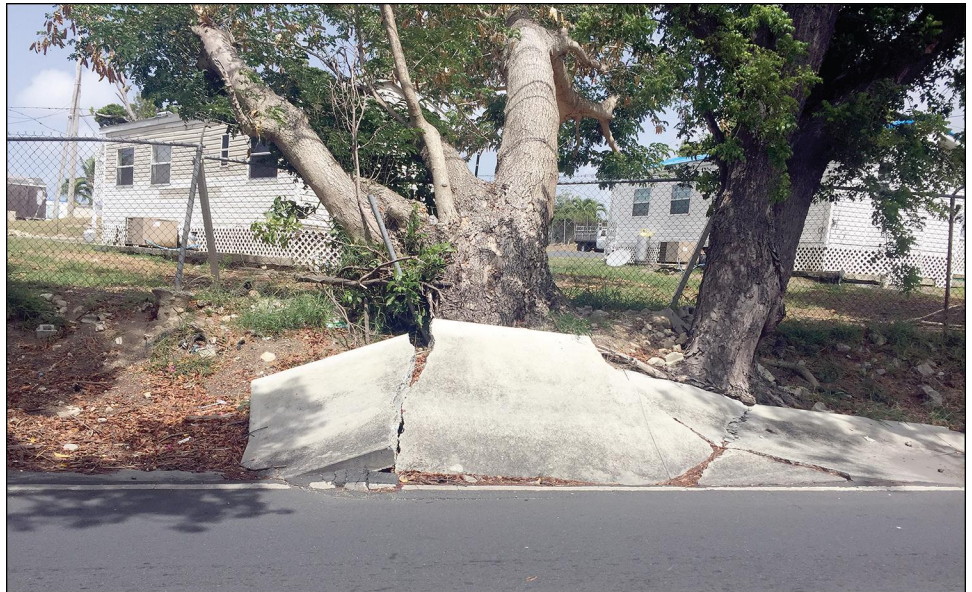
This sidewalk connected a busy bus stop to the island's only hospital.
