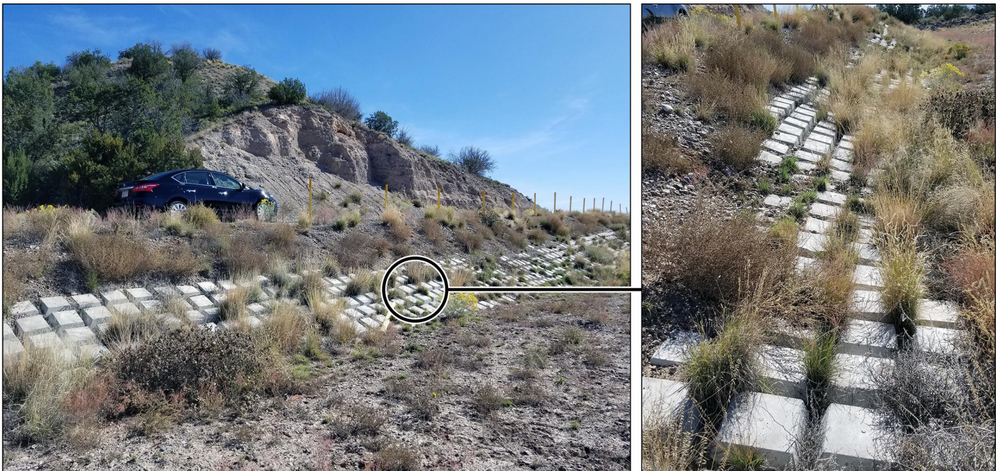
Figure 5: Example of Tribal Hazard Mitigation Project After a Flash Flood Washed Out a Road in 2013
